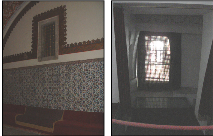
Figures 16a-b: Grilled window on the wall of the Court Hall, seen from the Court Hall and the Tower of Justice, photographed by the author
