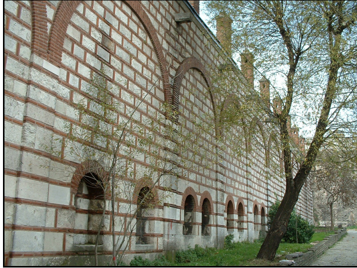
Figure 57: Restored exterior walls with alternate courses of brick and stone, Medrese, Edirnekapı Mihrimah Sultan Complex, photographed by the author
