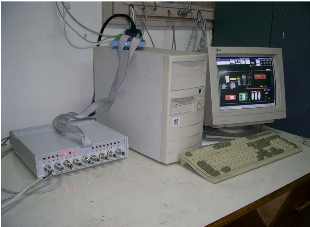
Figure 3.6.1: General view of control table.
