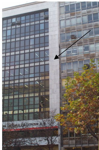
Figure III.102 Stone panels have been fixed with screws to the back up wall to prevent falling down (2004).
