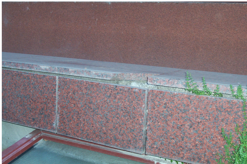
Figure III.93 Differential settlement has caused the detachment of stone panels from the fixing element and crumbling of the stone panels (2003).
