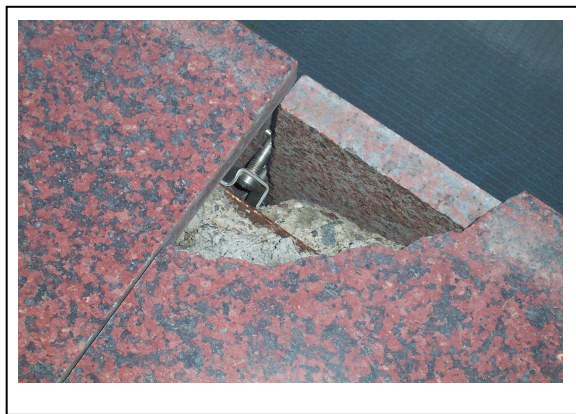
Figure III. 25 Stone crumbling. Ankara Kurtulus Park Wedding Ceremony Hall Parapet Wall. (2002)
