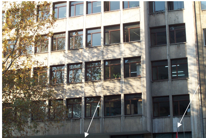
Figure III.64 Stone panels have fallen down and the whole façade stone panels have been screwed, Discoloration of the whole façade due to air pollution and wrong window sill detail. (2003)
