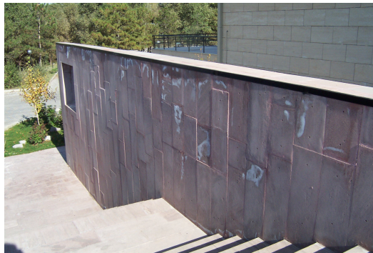
Figure III.99 The Ankara stone on the retaining wall has got wet and soluble salt in the mortar and stone has caused staining of the stone (2004)
