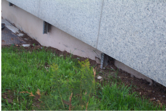
Figure III .106 Thermal insulation material does not continue under the fixing profiles of the curtain wall (2004).
