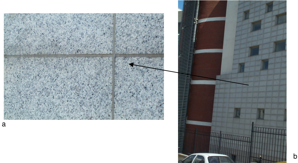
Figure III.105 Discoloration of stone panel joints (2004)
