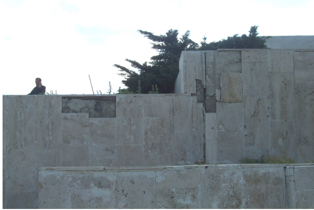
Figure III.84 Stone fall down at the construction joint of the retaining wall and the top of the wall due to water penetration under stone panels (2004)
