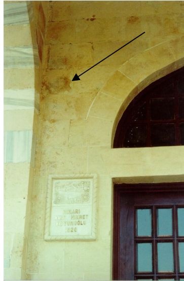
Figure III. 48 The brownish color of the travertine stone (2002).
