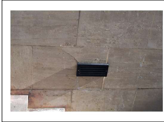
Figure III.26 Stone crack. METU Cultural & Conventional Center wall by the staircase. (2002)
