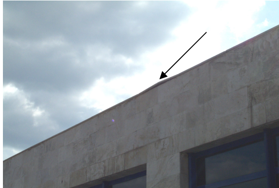
Figure III.76 Displacement of parapet wall coping (2004).
