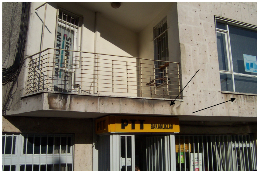
Figure III.72 Discoloration of stone under window sill and parapet wall copings (2002)
