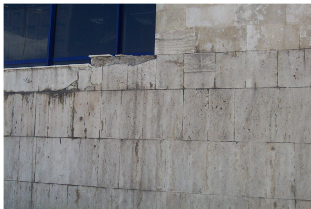
Figure III.77 Stone breakage and fall down due to the water penetration of the wall from the window sill. Some of the stone panels have been fixed by screws to the back-up wall. (2004).
