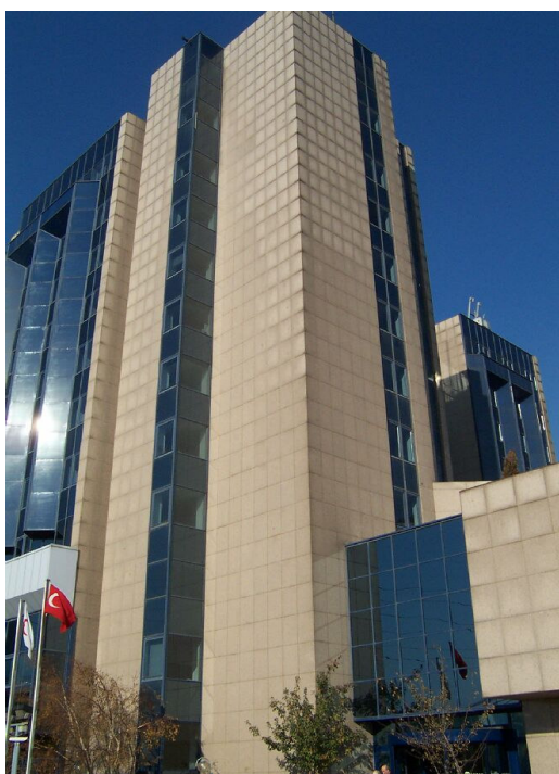
Figure III.91 Discoloration of the stone panel joints at the whole façade (2004)
