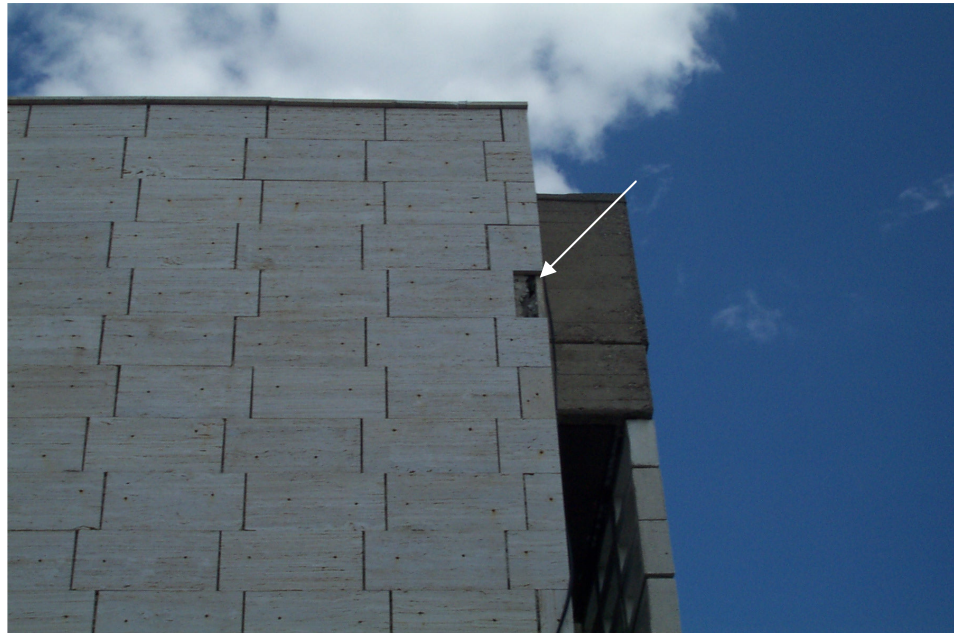
Figure III.69 Stone fall down at corner shows an irregular back structure and inadequate fill of mortar under stone panels. (2003)
