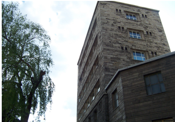
Figure III.60 Discoloration of stone cladding due to heavy traffic near the building.(2004)
