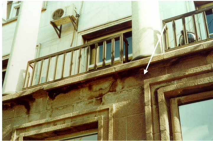
Figure III.51 White marble on the front surface is in a very good condition. Discoloration of the lower part due to the lack of waterproofing of the terrace (2002).
