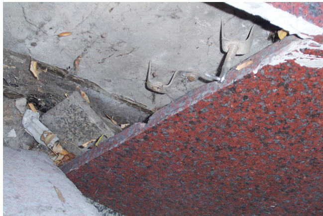
Figure III.94 The thickness of stone (2 cm) was not enough to compensate for the stress created by the dowel pin on the stone so it has broken and the adjacent stone panel displaced (2003)
