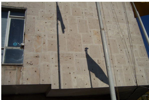
Figure III.71 All the stone panels were screwed after one of the panels had fallen down (2002)
