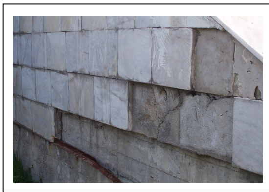
Figure III. 22 Stone fall down. Atatürk Cultural Center (May 2004)
