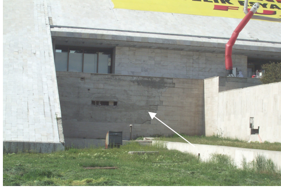
Figure III.87 Stone fall down due to improper water proofing of the horizontal surface (2004)
