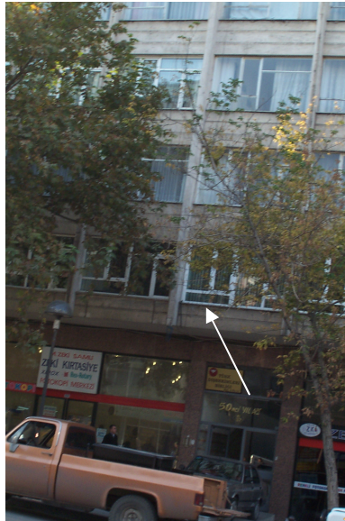
Figure III.66 All the stone panels have been screwed. The whole façade is discolored due to air pollution and water penetration under the window sill. ( 2003)
