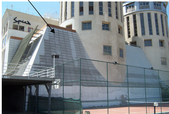
Figure III.104 Some parts of the sloped curtain wall are discolored but some are not ( 2004).
