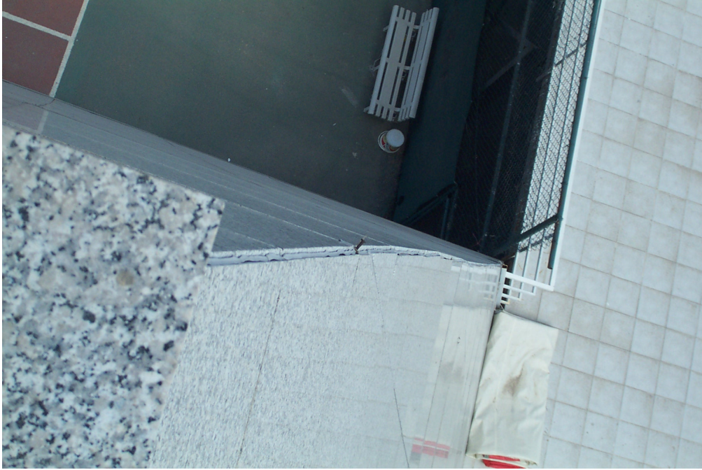
Figure III.110 Looking down from the terrace the slope stone curtain wall. The joint material has deteriorated and the cutting of the stone panels are not accurate .
