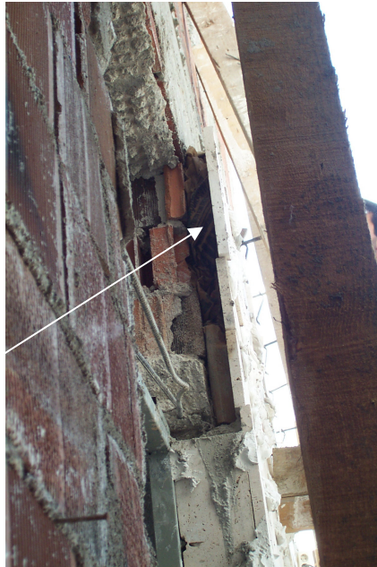
Figure III.78 Cement bags were filled into the back of the stone cladding wall during construction instead of mortar during the construction of the additional part of the building.
