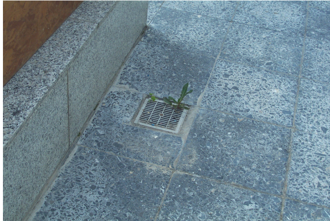
Figure III.108 The terrace on top of a sloped stone curtain wall. The vegetation is the evidence of continuously existing water under terrace tiles that can penetrate through the wall.(2004)
