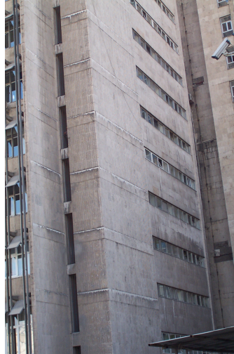
Figure III.75 Stone discoloration at storey cut profiles. Stone panels have been screwed against fall down. (2004)
