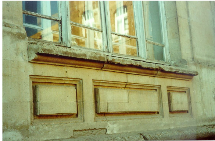
Figure III.45 Stone failure at window sill (2003).
