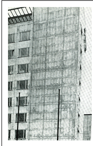
Figure III.17 Efflorescence due to soluble salts in grouting (Schaupp, 1967:62 ).
