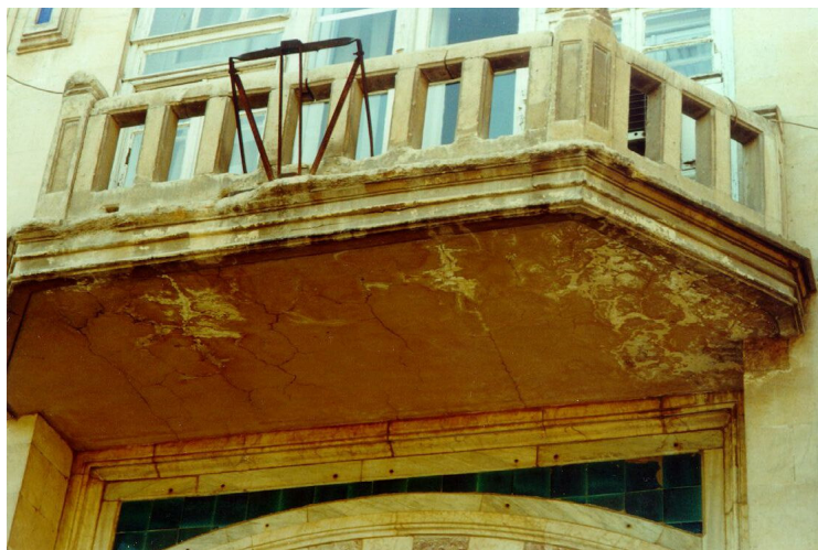
Figure III.46 Failure of stone elements under balcony (2003).
