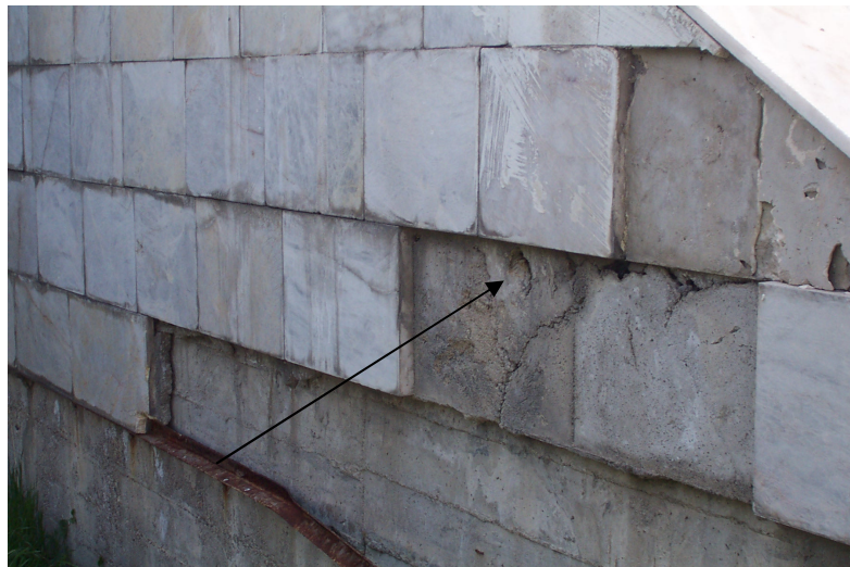
Figure III.83 Stone fall down due to irregular back structure and water penetration to the back of stone panels and corrosion of the fixing elements (2004)
