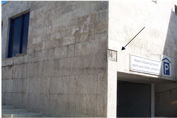
Figure III .74 Stone fall down at the corner due to a void at mortar behind the stone panel (2004).
