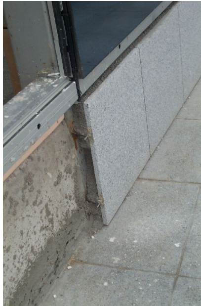
Figure III.113 There is not any thermal insulation material on the concrete wall. This may cause energy loss and condensation in time (2003)
