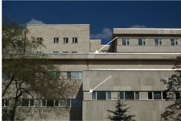
Figure III.58. The white travertine has been cleaned and some of stone panels close to the corner and the vertical expansion joints had fallen down and replaced with the ones that are different in color. (2004)
