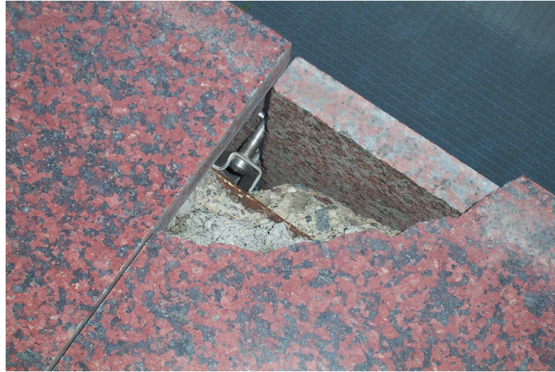
Figure III.95 The corroded metal element could cause stone crumbling. The back of the stone is empty, so the compression stone may cause breakage (2002)
