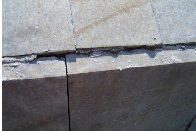
Figure III.82 Deterioration of the joint material (2004)
