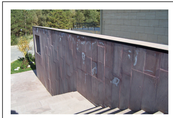
Figure III.27 Staining of the travertine stone. The METU Cultural & Conventional Center wall by the staircase.(2002)
