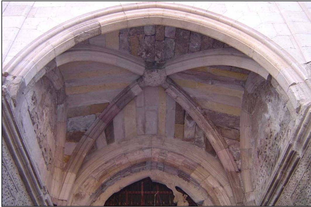
Figure 51 Sungur Bey Mosque- Ribbed Cross Vault of the East Portal (D. Esin)
