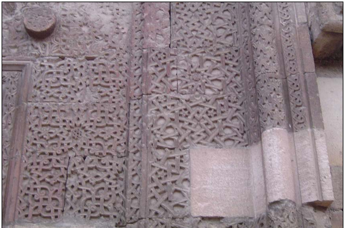
Figure 34 Sungur Bey Mosque- Detail from the Decoration of the North Portal (D. Esin)
