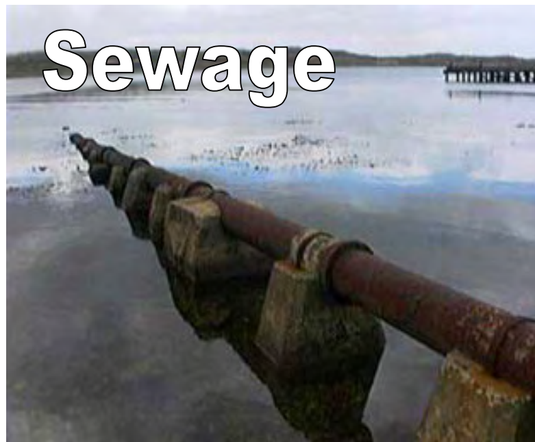
Figure 27. Evidence of Sewage
