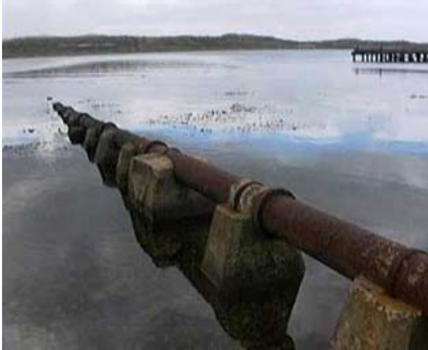
Figure 39. Evidence Of Sewage
