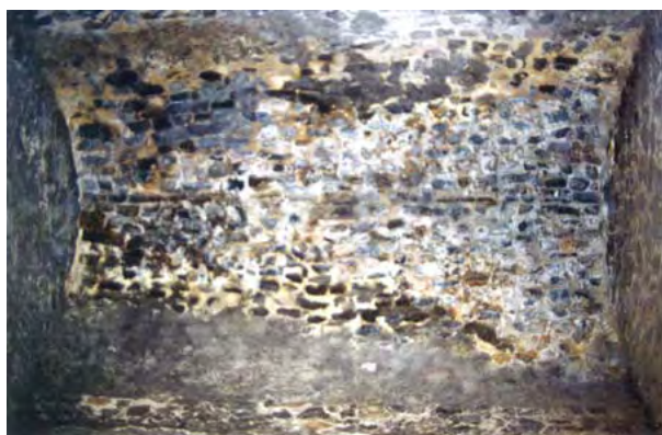
Fig. 4.40. Salination and black deposits problem on the vault of Space #9
