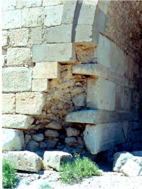
Fig. 4.21. Damaged wall corner next to Semi open space #3
