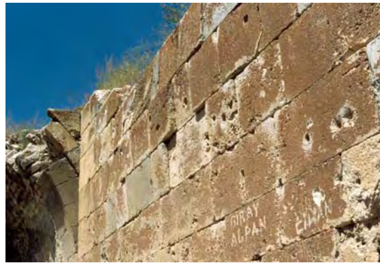
Fig. 4.38. Vertical detachment, bullet holes and lichen colonisation on the face stones of courtyard east elevation.
