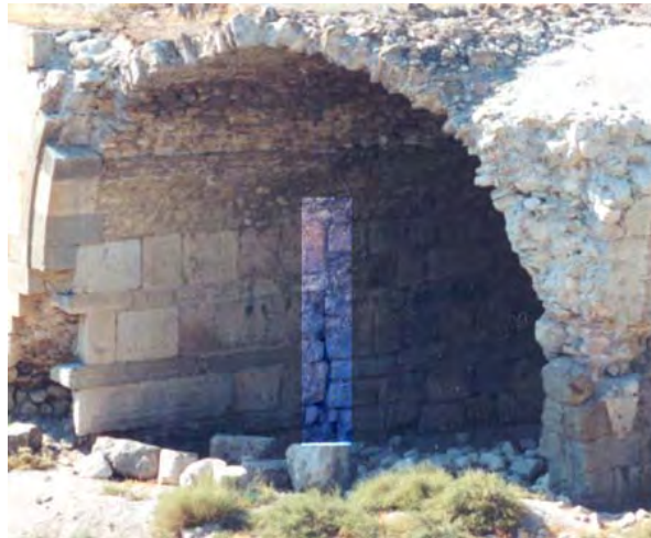
Fig. 4.22. Joint on the west wall of the first gallery of Semi-open space #3
