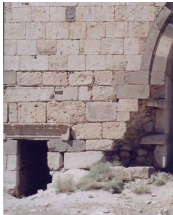
Fig. 3.26. Difference of workmanship on the north elevation of courtyard
