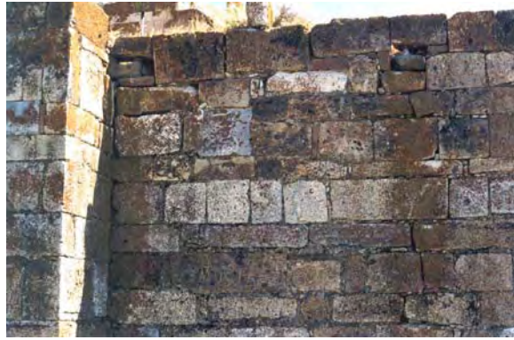
Fig. 4.42. Lichen colonisation below the water spouts on the north exterior elevation
