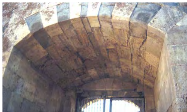
Fig. 4.39. Deterioration on the vault of Entrance Space due to the rainwater penetration
