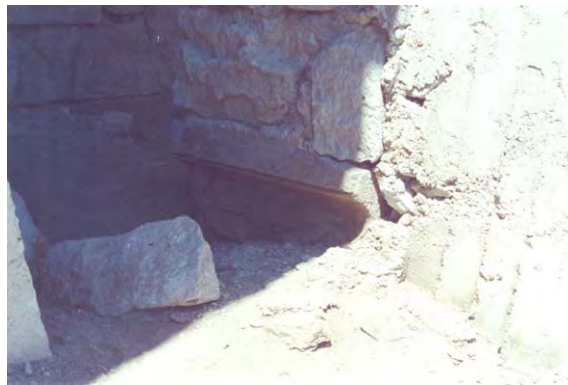
Fig. 4.43. Fallen piece of cornice combined with concrete repair
