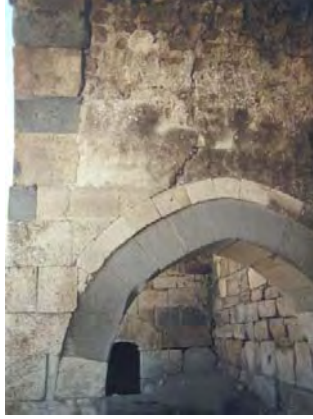
Fig. 3.39. Crack on the vault of Semi-open space #1
