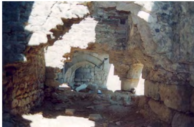
Fig. 3.37. Damaged south wall of Space #11
