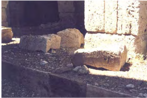
Fig. 4.31. Fallen pieces on the platforms located below the dome
