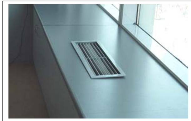
Figure 4.1. Fan Coil Units Located under the Glazing in Offices
